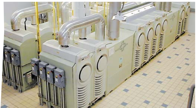
Overlooking the Capstone MicroTurbine installation at Harbec Plastics.
